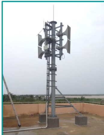
Alert Tower Digital Mobile Radio
